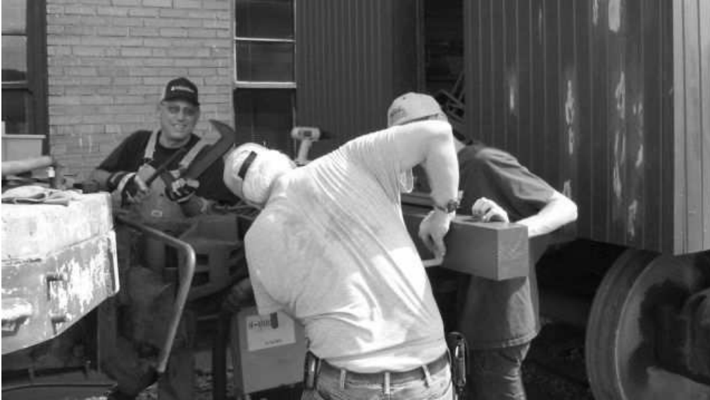
Steve Corp, Gale Meek and Rick Grosvenor are installing hardware on the north end sill of the Frisco caboose. Plans are to have both ends finished this year. This will complete the exterior work.
